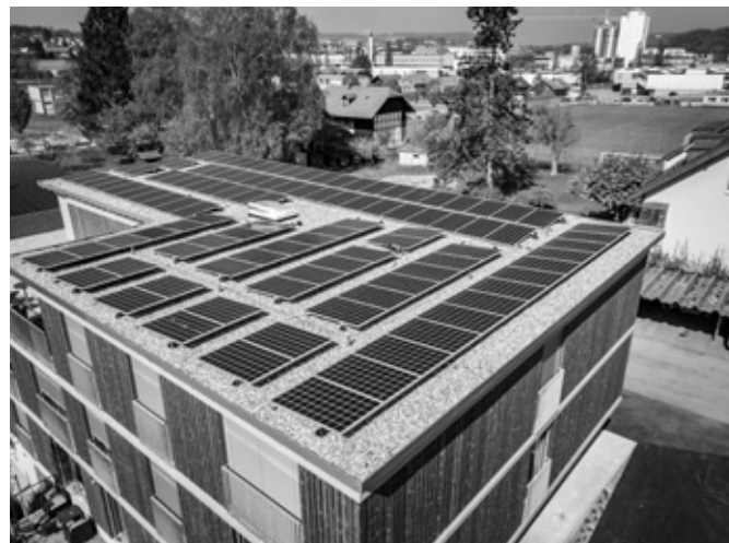
Photovoltaik Anlage (©Fengari AG)
